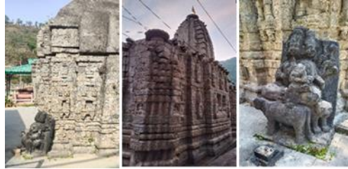
Fig. 9: Deteriorated Temples and Sculptures
