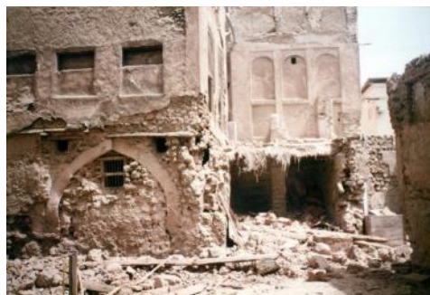
Fig. 4: Limestone walls and palm mat roofing details - Bait Al O'oud, 2010, during the demolition of the house.
