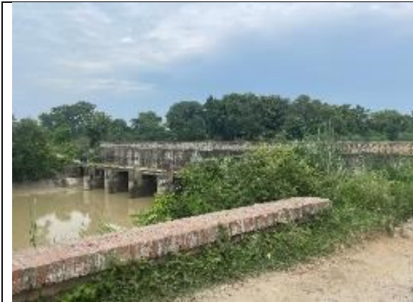
Fig. 21: Canal passing below Putri river in Ranipur. Source: Authors, 2024
