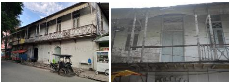
Fig. 6: Damage to WB Ledebour & co building. Source: photograph by Author 2021
