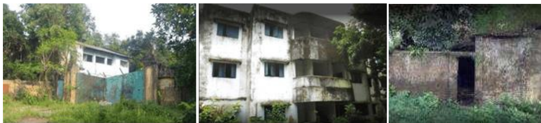
Fig. 18: Housing (good conditioned, partially damaged and fully damaged from left to right respectively)
