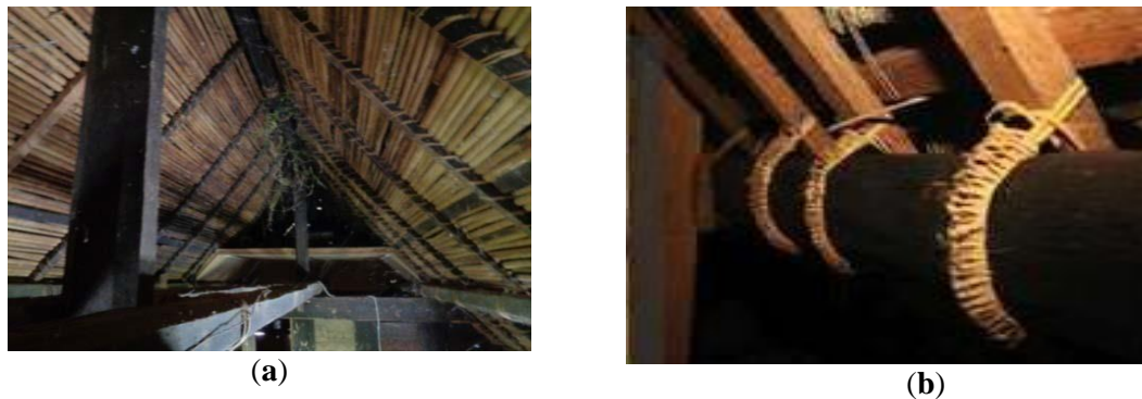
Fig. 3: Clamp and binding joint technique in roof part: (a) Clamp technique in roof part; (b) Binding joint technique in roof part
