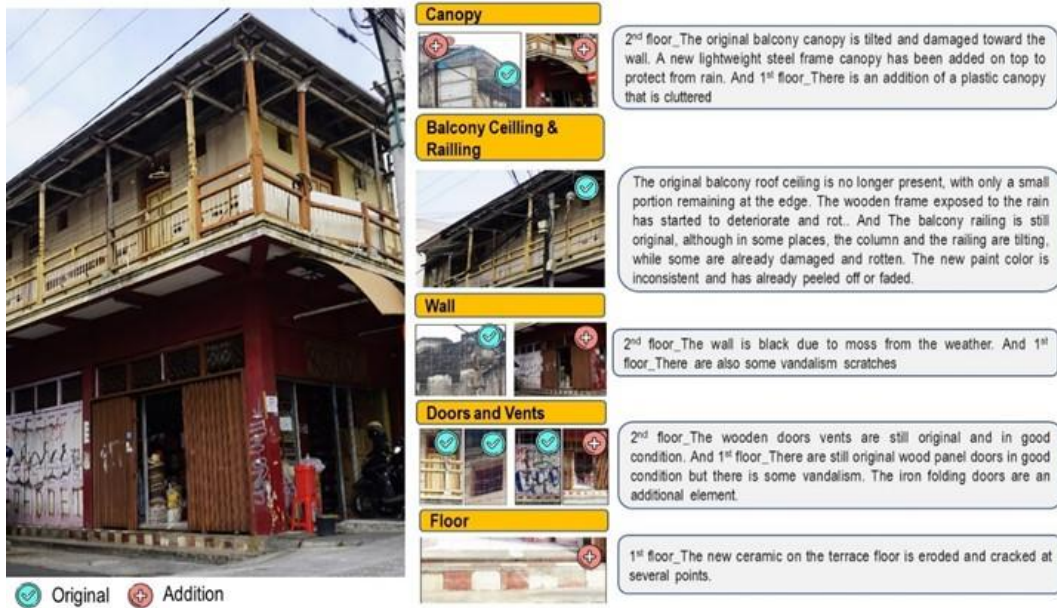
Fig. 18: Identification of Facade Damage of the Windiastuti Shop House Source: Author, 2023
