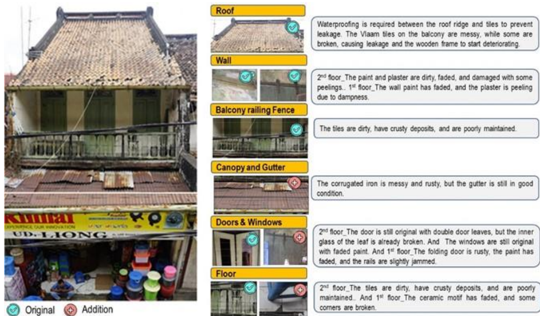
Fig. 15: Identification of Facade Damage of the Liong Shop House Source: Author, 2023
