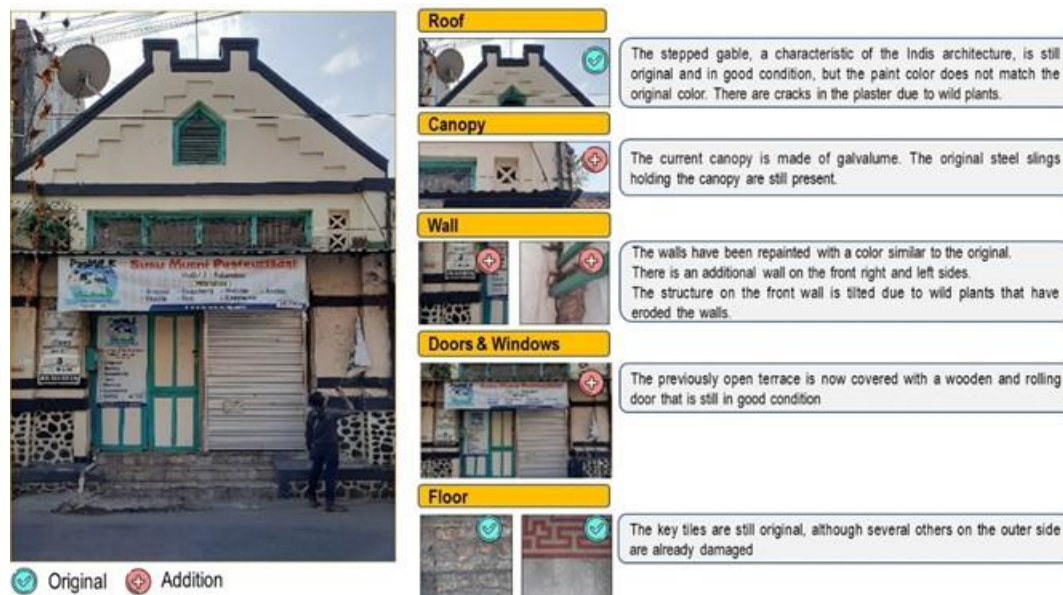
Fig. 7: Identification of Facade Damage of the Kwan Nio Tio Shop House
