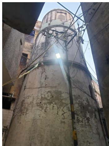
Fig. 12: Deterioration of the structure.
