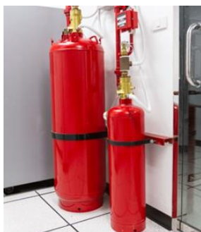
Fig.8: Novec 1230 Fire Suppression
