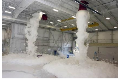
Fig.5 Automatic Foam System
