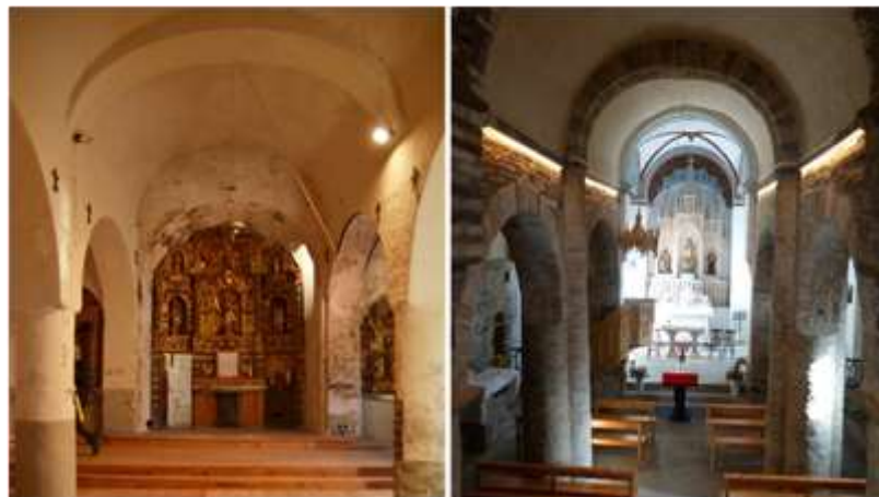
Fig. 4. Deformations in the churches of Santa Eularia d'Unha and Santa Maria de Vilamós. Source: Author
