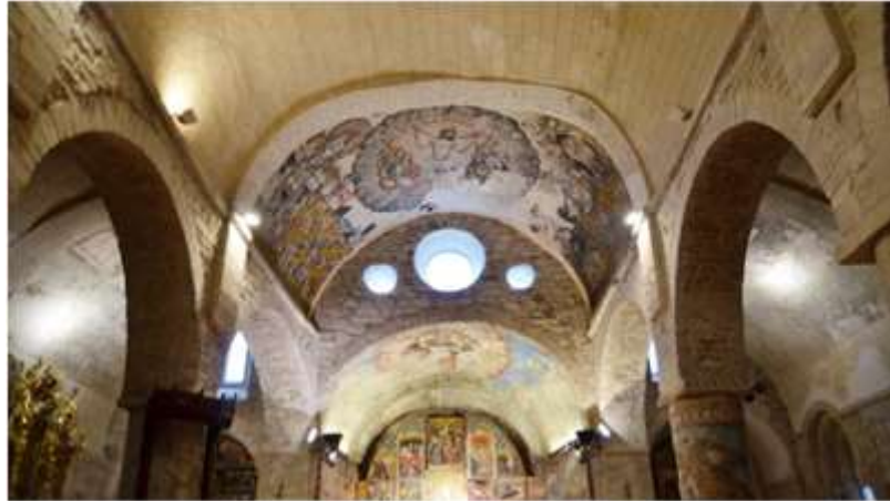
Fig. 5. Large deformations in the church of Santa Maria d'Arties.
