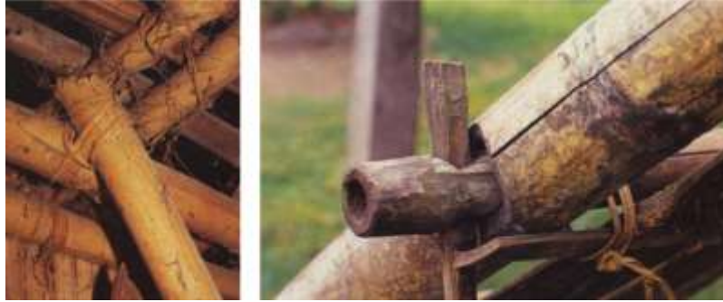
Fig. 8: Typical Joinery details of bamboo commonly seen in the North East: Bamboo Tie with Cane Ropes (left) and Dowel & Tenon Joint (right).
