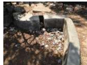
Fig. 30: Lack of awareness leading to disruption of rain water drains. Image showing a garbage dump at one such drain. Source Author
