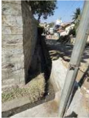
Fig. 23: Traditional stone pipelines placed along the road to channelize rain water runoff to the water tanks.
