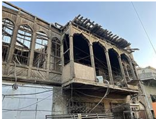
Fig. 1: Wooden elements in a dilapidated traditional Baghdadi house Source: Authors, 2023
