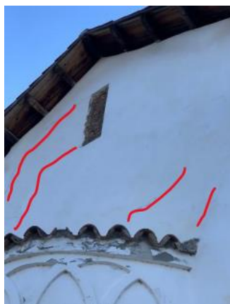
Fig. 3: Cracked masonry wall above the apse Source: Author
