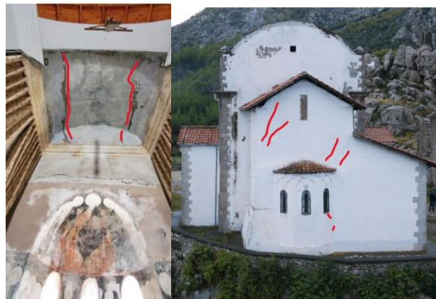
Fig. 5: Cracks in the vault of the apse and the wall Source: photos were taken by the author
