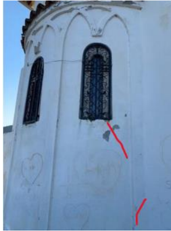
Fig. 4: Micro cracks in the wall of the apse Source: Author
