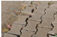
INADEQUATE WALKING SURFACE
