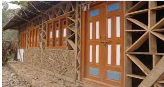
Fig. 4: Dhajji Diwari Construction in Himalayan Region of Kashmir Source: UN habitat and SDC.
