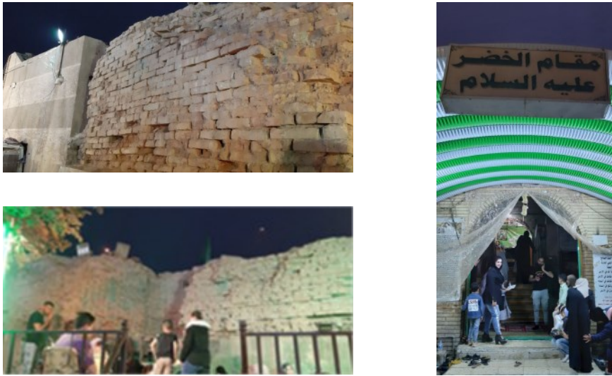
Fig. 7: The poor constructional situation of the shrine as it appears in the side elevations, as well as the poor and temporal additions to the entrance.
