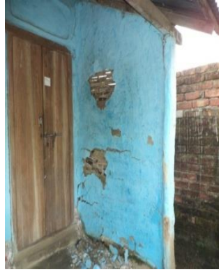
Fig. 4: Wall damage in house type BBGI1LNG Source: Author
