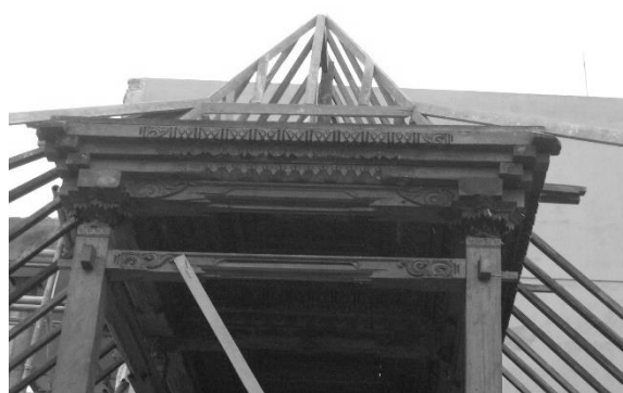
Fig. 5. The roof rested on a series of beams ( blandar and pengeret ) placed at the ends of saka (pillars)
