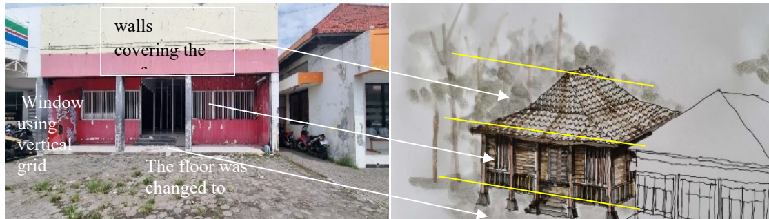
Fig. 10: (a) The building of the former official residence of the post office head changes to the front view, the stilt floor that has been lost. The interior of the building remains in good condition; (b) A sketch of the former official residence building is still visible in 2004 Source: field survey in 2004 and 2022
