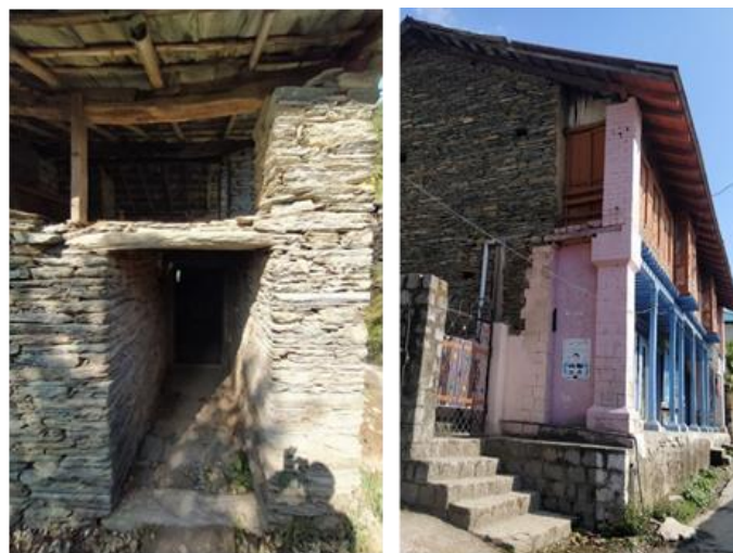
Fig. 11: 600mm Stone Column (left) and RC Column to support larger span (Right) Source: Author
