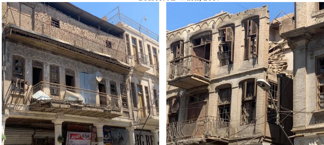
Fig. 6: The disintegration of old buildings, many of which were removed as a result of the Baghdad Municipality's neglect of the decision issued in 2009 to develop Al-Rasheed Street.
