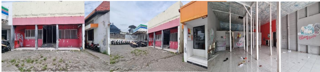
Fig. 9: The rest of the stilt building, the stilt floor, was replaced with ceramics. Meanwhile, the interior, such as the pillars, walls, roof, and ceiling, is still intact: survey 2022
