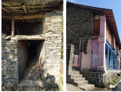
Fig. 11: 600mm Stone Column (left) and RC Column to support larger span (Right) Source: Author,2022
